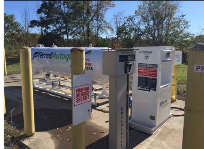
Autogas Dispenser, 1000gal Tank & FMS Tower
